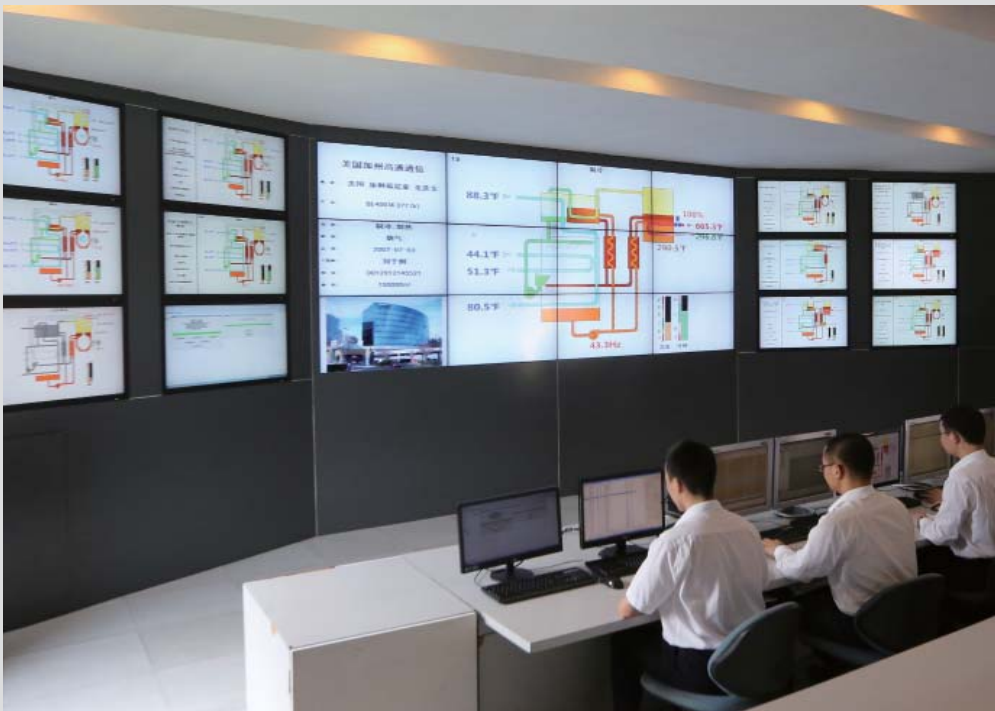
Global Internet Monitoring Center for BROAD central air conditioning. It has been operating since 1996, known as the pioneer of "internet +".
