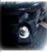
Anti-vibration pad of fan motor
